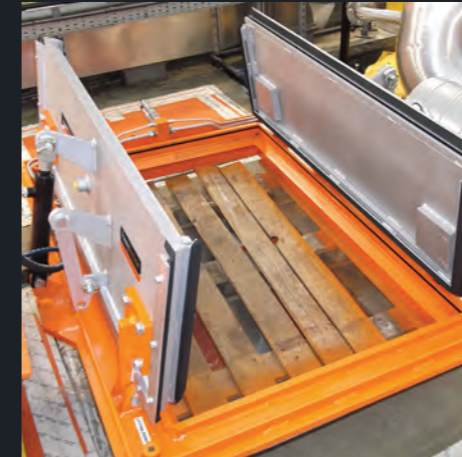
Bradwell hydraulic shield doors
