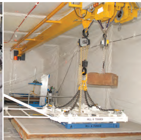
Sellafield cell cover lifting frame
